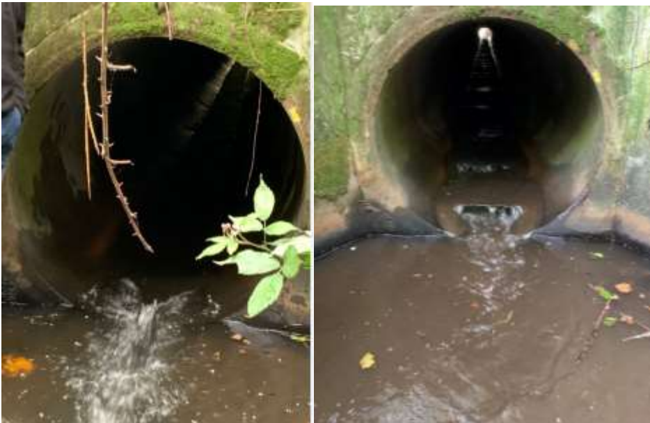
Figure 6: Culvert remediations in a tributary of the Mangawhero Stream, Ohakune. Flexi-baffles were installed throughout with mussel rope (top right) attached to the apron of one culvert to allow climbing species to pass.
